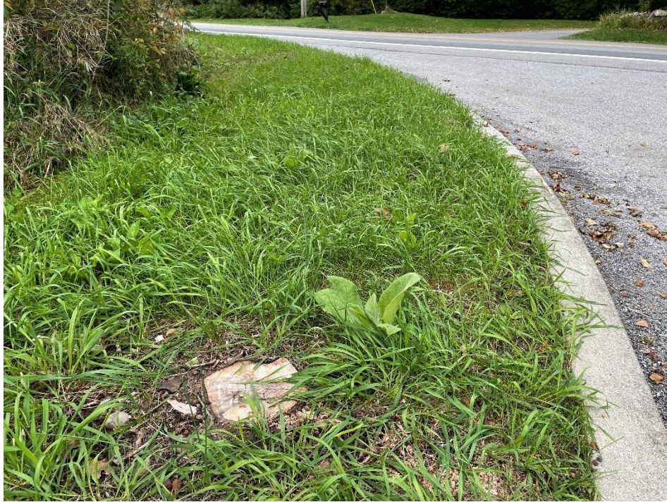
Curb cut had 15 years of tree and brush growth. Removed this summer and now in grass.
